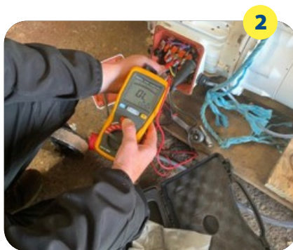
Taking insulation readings from motor windings.
